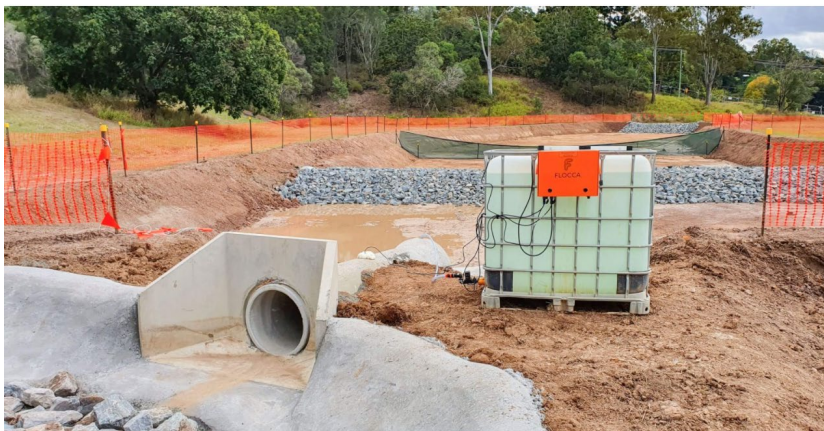
Image 2. Illustrates a filtering drainage (floccla) system installed on the Songbird Oxley site. adopting a flow based automated dosing unit which accurately doses chemicals to treat collected water on site. The system improves finished water quality prior to discharging offsite.
